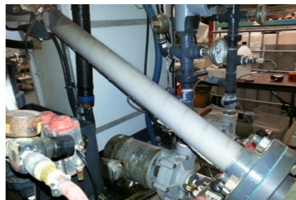
Solids extraction system
