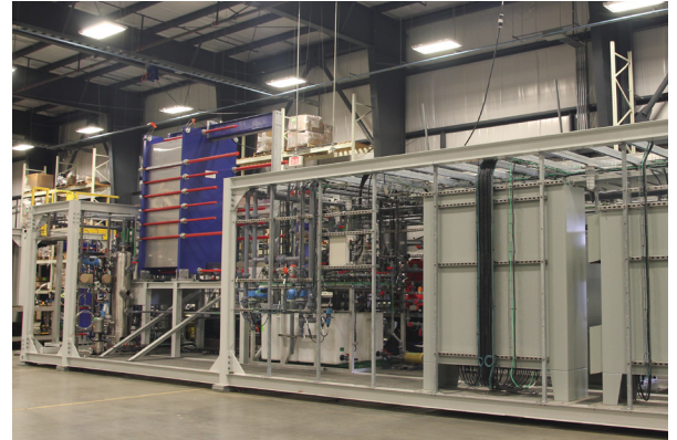
A SaltMaker MVR plant being assembled
