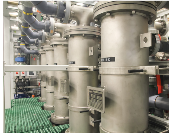
Membrane vessels in an XtremeUF plant
