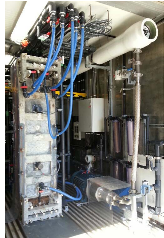
Saltworks' EDR-RO hybrid system
