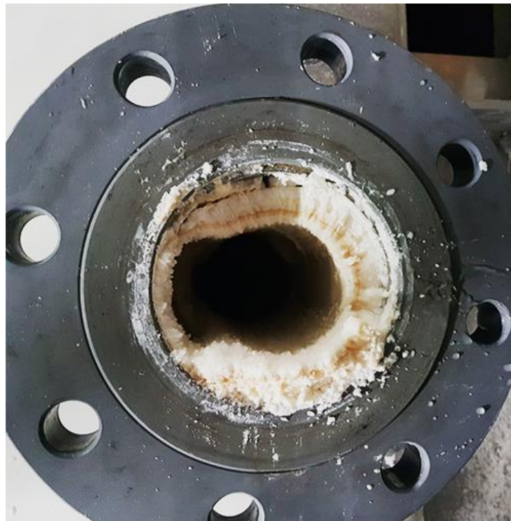
Scaling in a pipe
