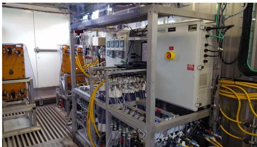
Fig 10. Flex EDR Ammonia pilot plant
