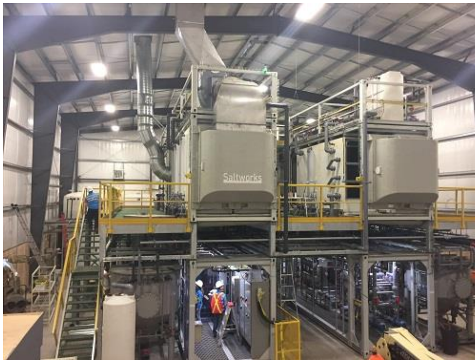
SaltMaker Evaporator Crystallizer Installed at BC Site
