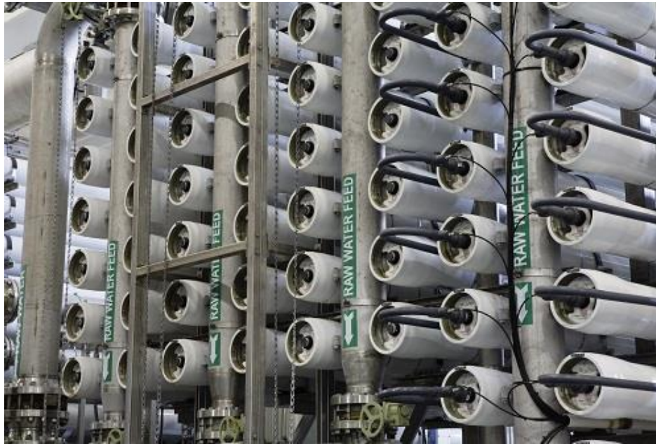
Membrane Treatment Systems
