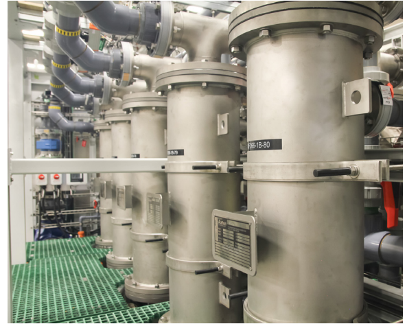
Membrane vessels in an XtremeUF plant
